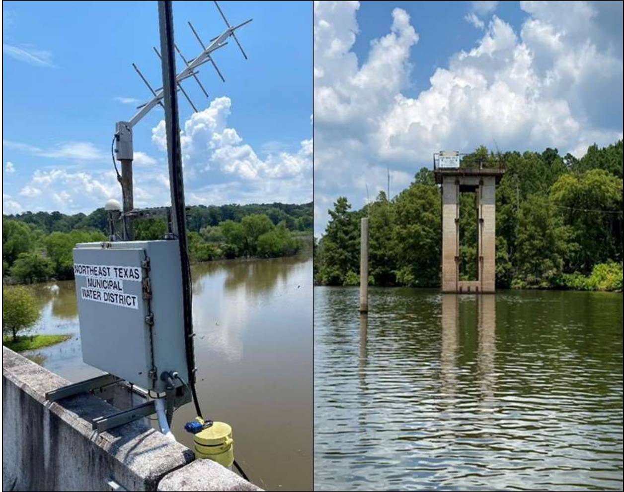
Figure 15: Continuous Water Quality Monitoring Stations; US 259 (left) and NETMWD Intake (right)
