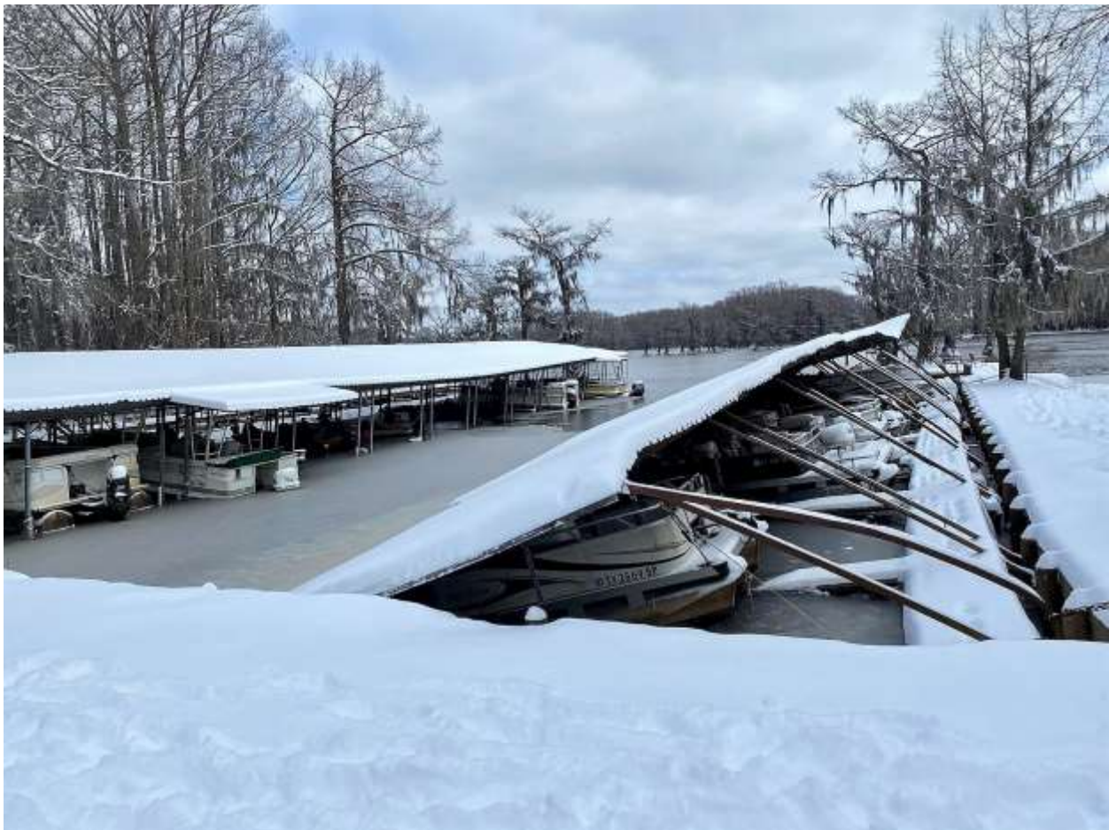
Figure 49: Damage caused by the February 2021 winter storm at a marina on Caddo Lake
